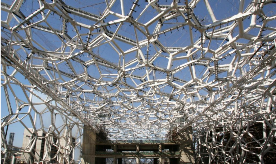
Fig.4.14 – Interior view of the Water Cube pavilion showing the almost complete structure (source: (Eastman, et al., 2008))
