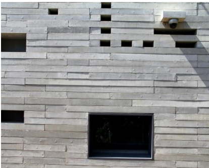
Fig.7.6 - An image of the facade, where it is visible the concrete slabs with different sizes and the produced empty spaces (source: http://guedescruzarquitecto.wix.com/pt )
